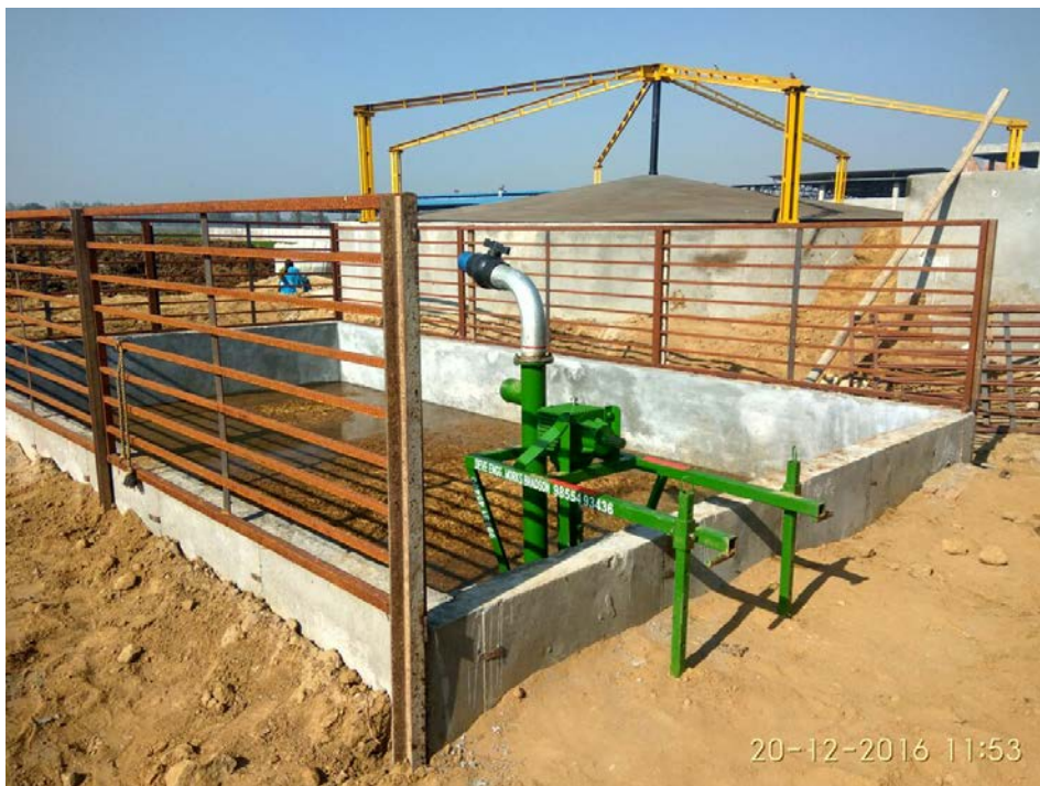
MIXING TANK WITH STIRRER AND FEEDING PUMP
