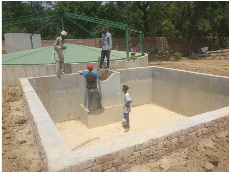
DIGESTED SLURRY EVACUATION TANK WITH PUMP
